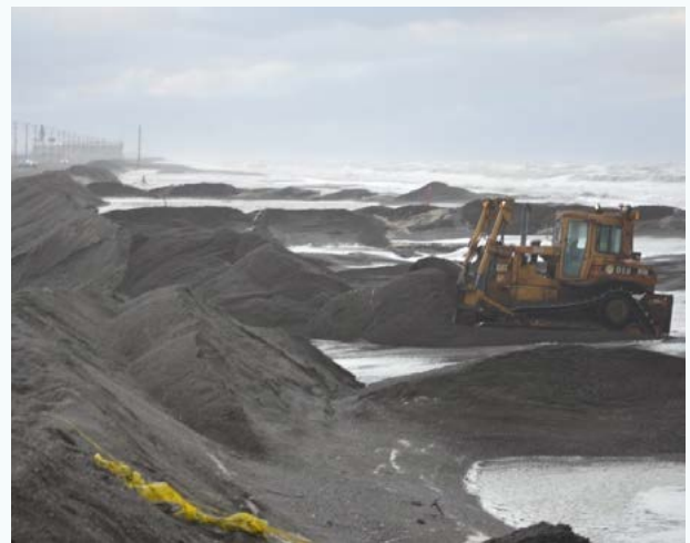
Figure 42: A five mile gravel berm provides insufficient shoreline protection from coastal erosion in Utqiagvik and must be repaired after every storm, as shown above, which costs $8.3 million annually. The U.S. Army Corps of Engineers project will construct a fortified rock revetment to protect the shoreline. Credit: North Slope Borough.
