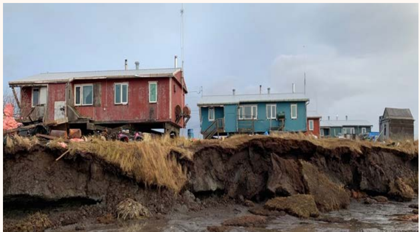
Figure 16: The eroding riverbank (shown above in 2018) forced Newtok to demolish these homes in 2019 to prevent them from collapsing into the river. Credit: John, Andrew; Village of Newtok; 2018.
