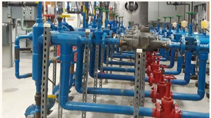
Figure 25: Thawing permafrost in Noatak caused a crack in the floor of the water treatment plant and the foundation has settled significantly resulting in threats to the integrity of the pipe system. Credit: ANTHC.
